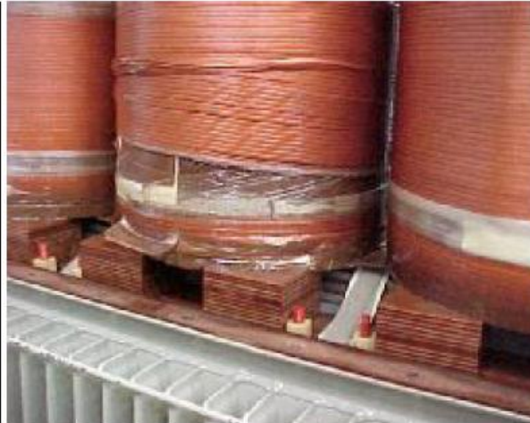
Fig.4 Primary windings of distribution transformer after a failure.
